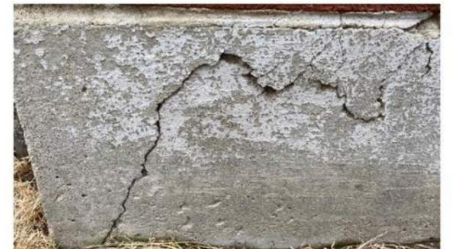
Cracking foundations and uneven settlement.
